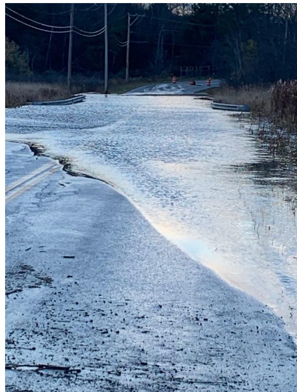
Figure 2. Flooding along Hollow Road, Monkton, VT in November 2019
