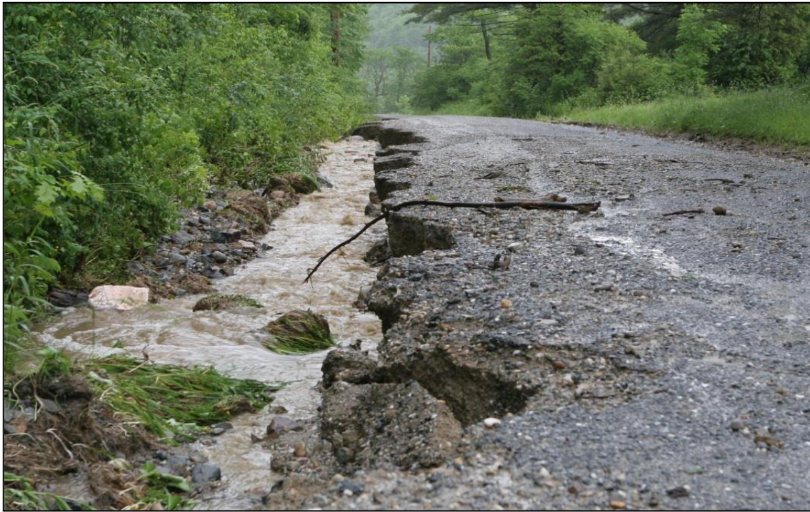
Stormwater degrades a Monkton Road Photo credit: Buzz Kuhns.
