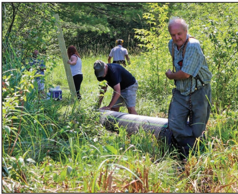
LEE KAUPILLA, RIGHT, and John Lavigne haul part of an 80-foot-long culvert pipe through the woods and marsh around Monkton Pond last month. The pipe now helps keep the water level in the pond constant by emptying water through a beaver dam.
