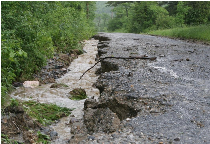
Stormwater degrades a Monkton road
